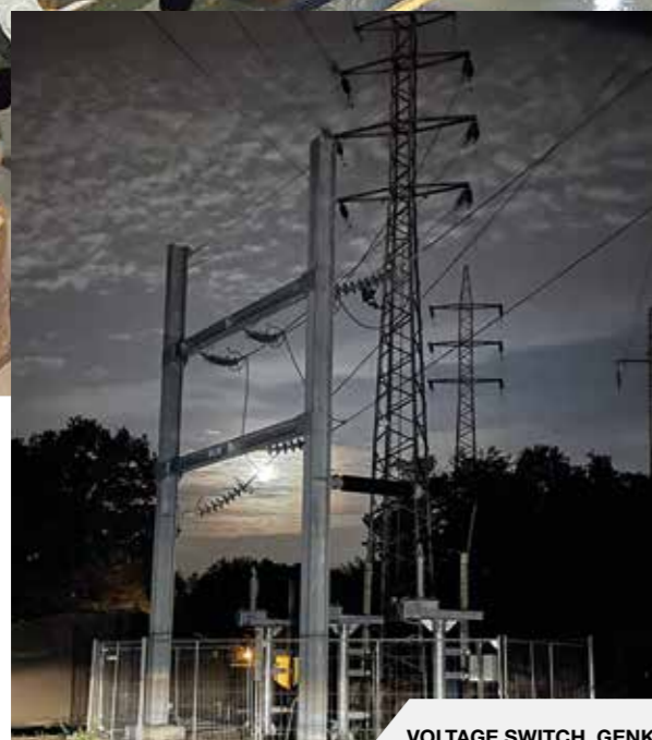
VOLTAGE SWITCH, GENK
