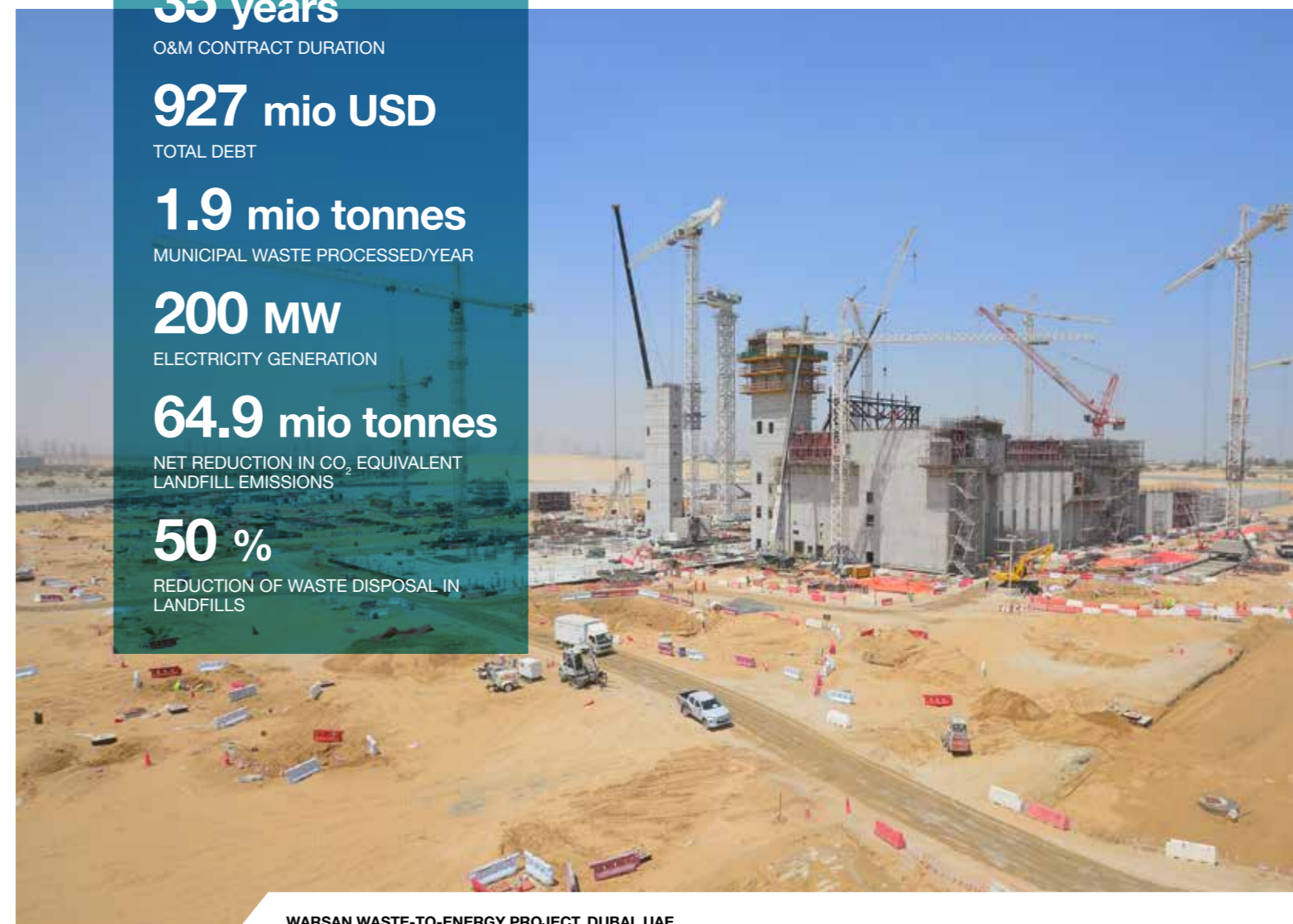
WARSAN WASTE-TO-ENERGY PROJECT, DUBAI, UAE
